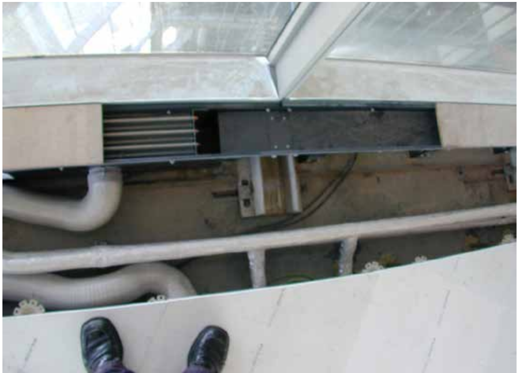
FIG. 3.6 Posttower Bonn – inner path of the double façade with service components (image: U. Knaack)
