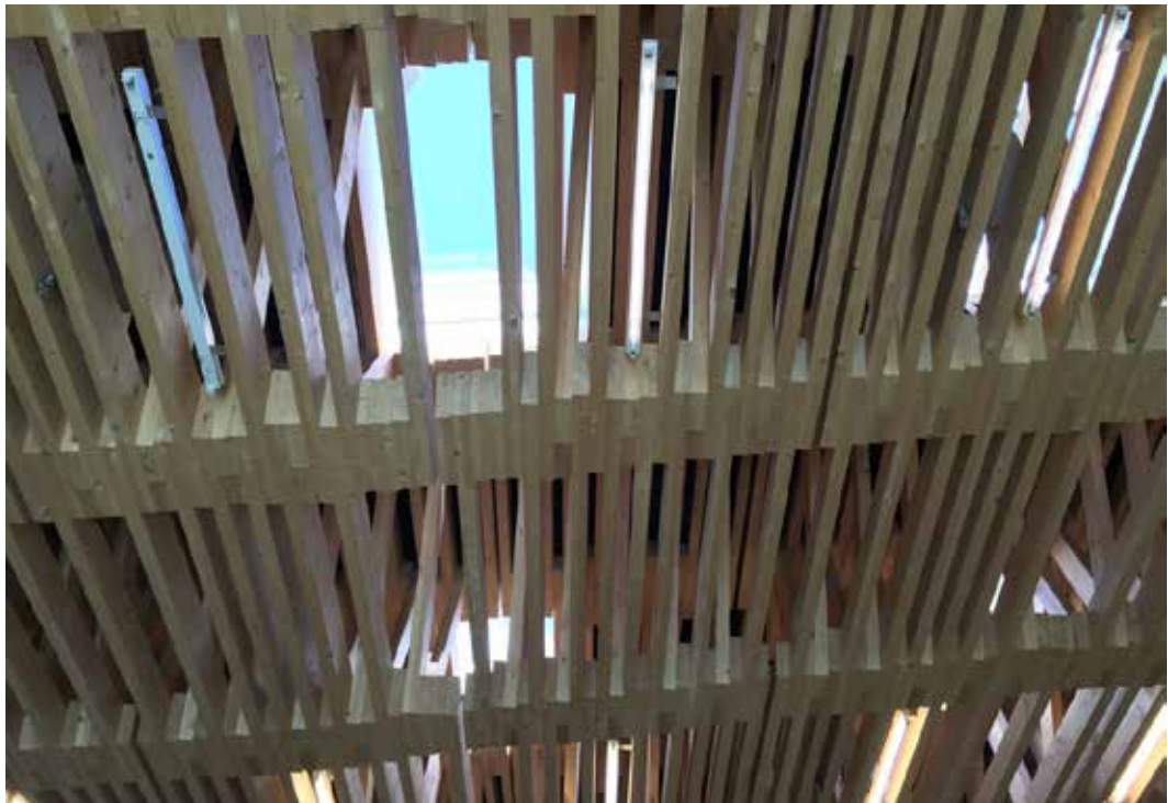
FIG. 2.5 The sequential wooden roof construction of the Arch_Tec_Lab building at ETH Zürich demonstrates the work of the hosted ITA-Institute: all design, dimensioning and fabrication processes were done consequently digitally and the assembly in 2016 was done by a roboter. (image: U. Pottgiesser)
