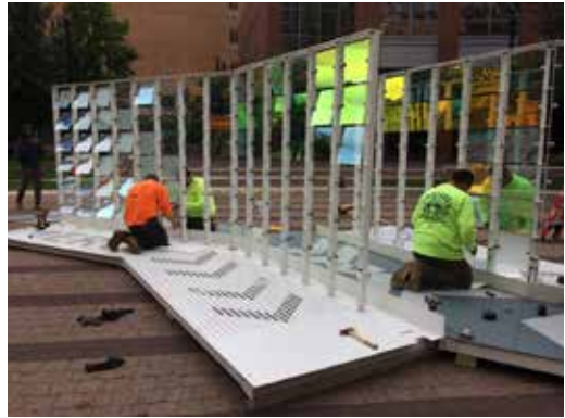
FIG. 2.10 Merge installation in Philadelphia showing architecture students and glaziers on site assembling the components of a multidisciplinary project. (image: J. Doerfler)
