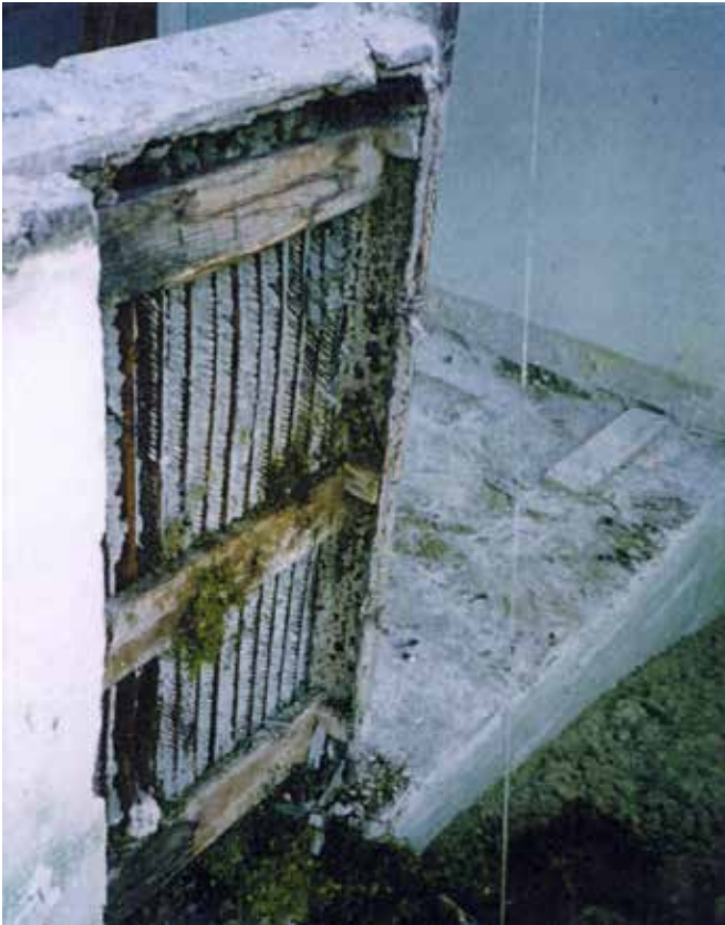
FIG. 5.9 'Destructive research' of an original part of the spandrel revealed wooden battens horizontally applied to the metal lattice (labelled as 'lath' in FIG. 5.7), which were not documented in any of the original drawings / Wessel de Jonge Architects
