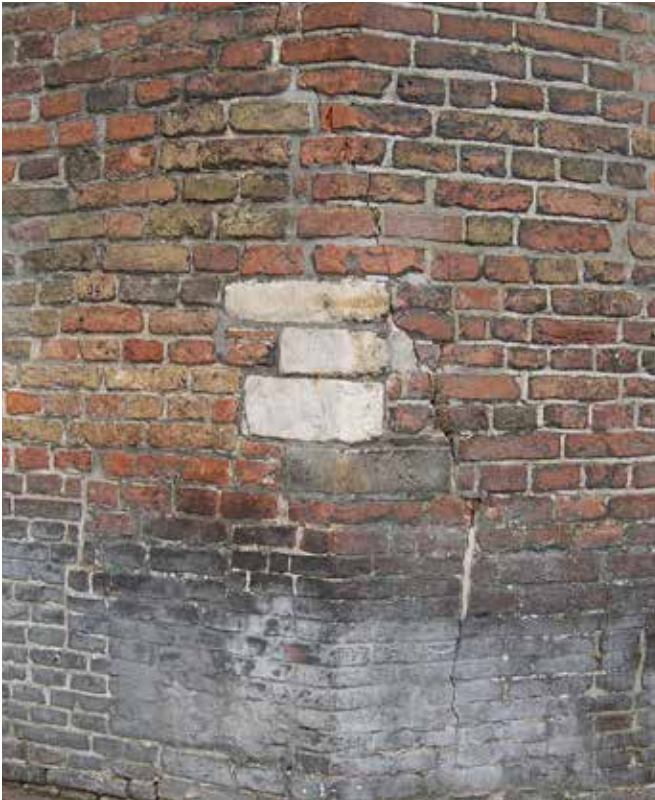
FIG. 3.15 Visible layers of repair in the wall of the medieval St Anthonis Gate, later reused as weigh house and place to demonstrate skills of brick laying for the guilds, Amsterdam / Marieke Kuipers
