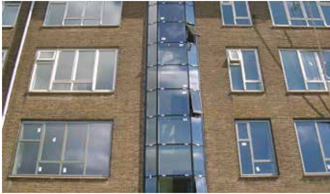
FIG. 4.9 Central part of the façade of the AWW social housing block at Landlust, Amsterdam, originally designed by Gerrit Versteeg and renamed as 'King's Wives', with new stairwell window frames being installed during the renovation to the design of Archivolt Architects / Marieke Kuipers
