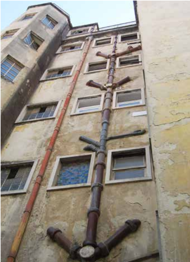
FIG. 3.39 External sewage pipes on a building in the old Carmo district of Lisbon / Marieke Kuipers
