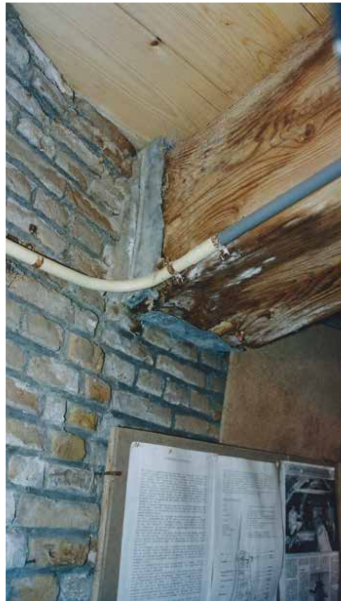
FIG. 6.13 Timber beam in an external wall, showing rot even though it seems well protected by the lead; NB this underlines that drying, which is in this case very difficult, is the most important issue in order to prevent moisture problems from becoming severe (windmill, Stavenisse, the Netherlands) / photo: R. v. Hees
