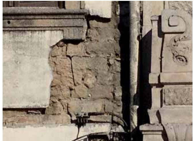
FIG. 2.18 Detail of façade constructed in local adobe and finished with a lime render (houses, Aveiro, Portugal) / photo: R.v.Hees
