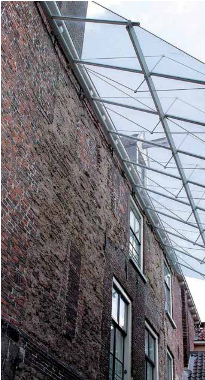
FIG. 6.3 Transparent roof construction as a protection for the tuffstone in the historic wall (house, Sandrasteeg, Deventer, The Netherlands) / photo: R. v. Hees
