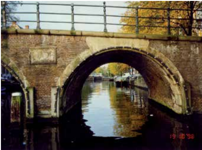
FIG. 7.2 Self-healing in lime mortar (canal bridge in Amsterdam, The Netherlands) / photo: R. v. Hees
