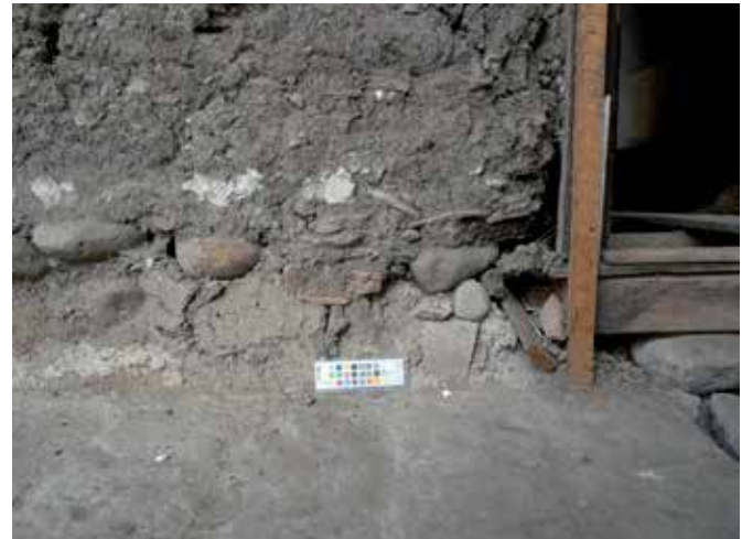
FIG. 2.11 Rubble stone masonry is used at the ground level to minimize the effect of splash-up (building in Cuenca, Ecuador) / photo: R. v. Hees
