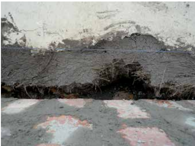
FIG. 2.13 Use of adobe for renders in a recent restoration (2010) (building in Cuenca, Ecuador) / photo: R.v. Hees
