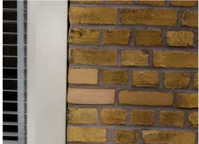
FIG. 6.17 Detail of wall with new bricks (house, Justus van Effen complex, Rotterdam, The Netherlands) / photo: S. Naldini
