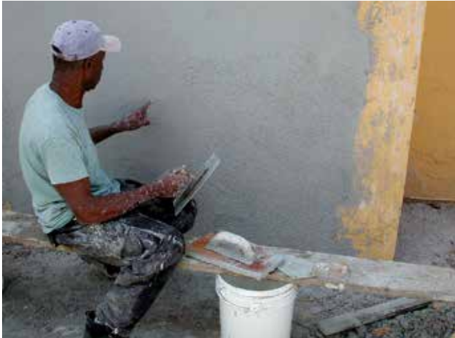
FIG. 4.13 Newly designed render compositions with assumed better salt resistant behaviour (house at Charloo, Curaçao, Caribbean) / photo: R. v. Hees
