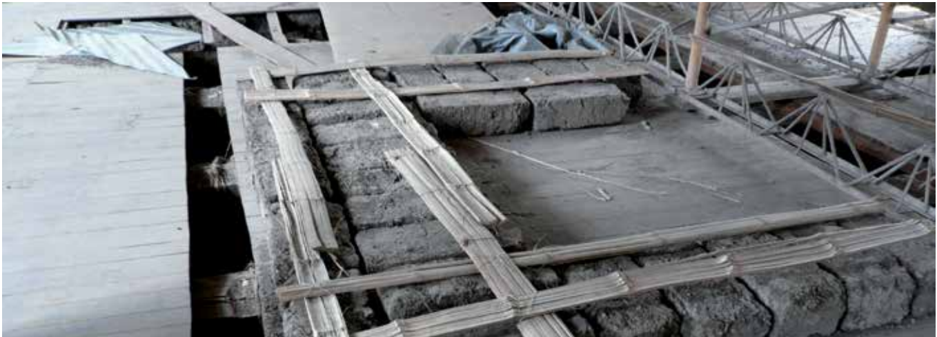
FIG. 3.9 Bamboo ready to be used as a ductile reinforcement in adobe walls (school building, Cuenca, Ecuador) / photo: R. v. Hees
