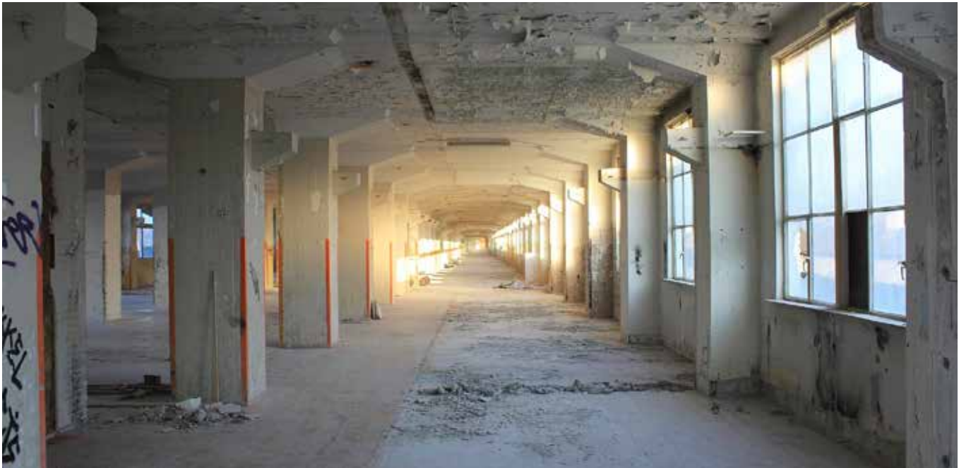
FIG. 7.11 View of the interior: essential and unrefined spaces (Sphinx factory , Maastricht, The Netherlands) / photo: Braaksma & Roos
