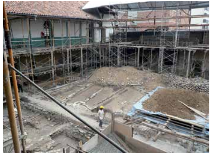
FIG. 2.9 Use of adobe in a restoration in Cuenca. The old material of a collapsed wing of the building is collected for re-use (house in Cuenca, Ecuador) / photo: R. v. Hees
