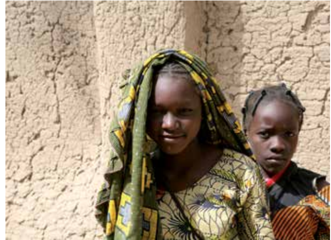
FIG. 2.6 Crack patterns, like crazing, can easily occur in the adobe rendering of external walls (Mali, Africa) / photo: L. Edelbroek
