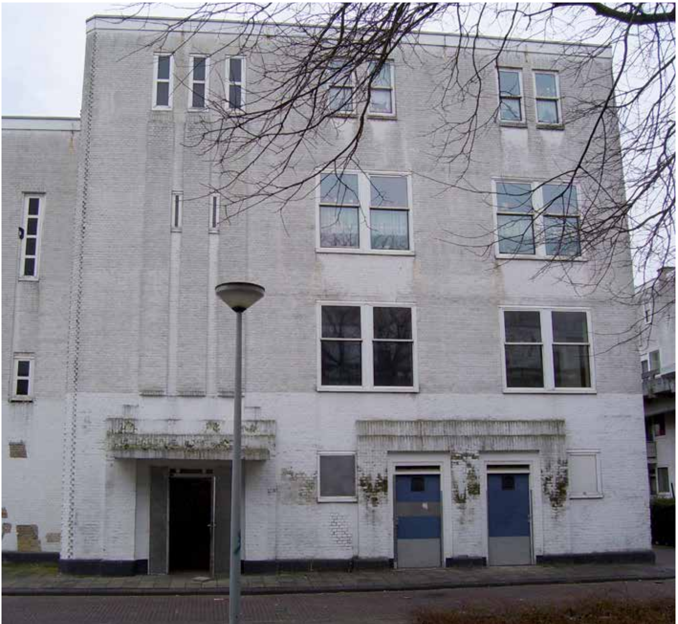
FIG. 6.15 Façade of one building showing damage (2009); to the left: paint removal - try out (Justus van Effen complex, Rotterdam, The Netherlands) / photo: A. Acquebord
