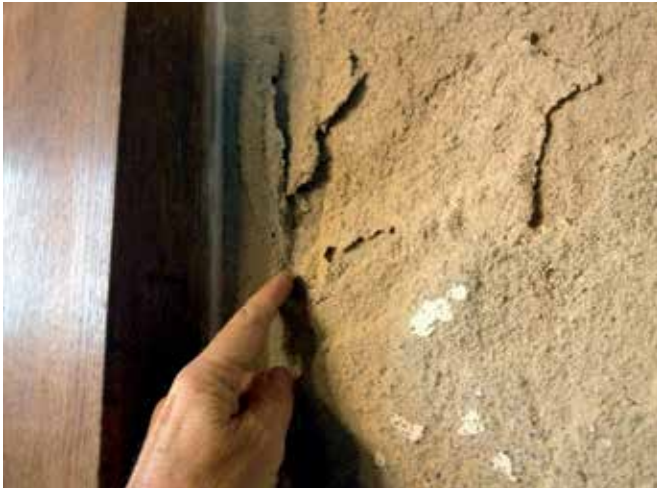
FIG. 7.4 Exfoliation and crumbling of plaster applied on a salt loaded substrate / photo: R. v. Hees
