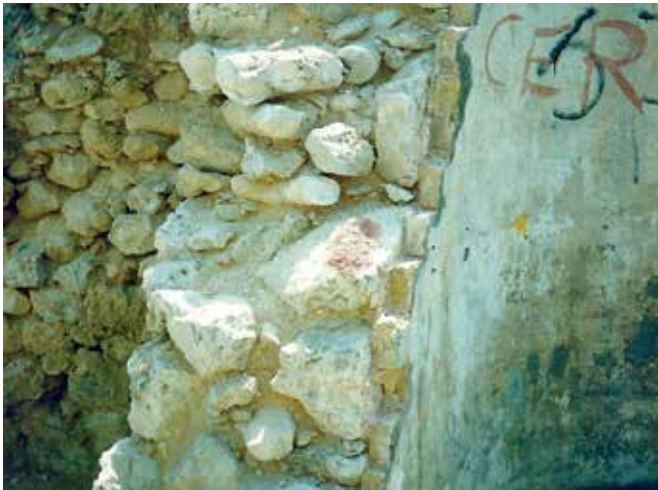
FIG. 4.3 Composition of a cistern wall: coral stone wall construction with an internal cladding of 'Jssel clinkers' and a two or three layer render system on the inside (Curaçao, Caribbean) / photo: R. v. Hees
