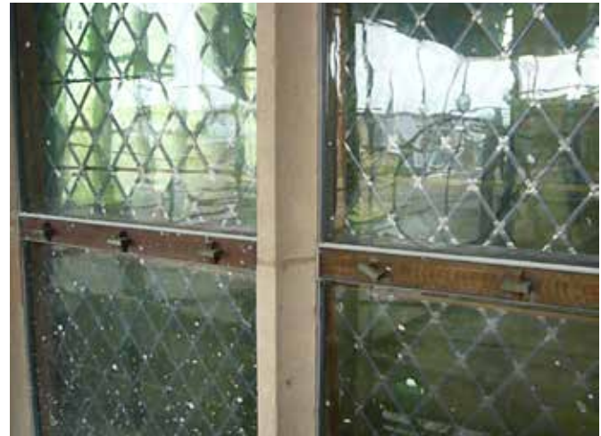
FIG. 6.6 Test panels for external glazing in front of the stained-glass windows (Peter's church, Leiden, The Netherlands) / photo: R. v. Hees
