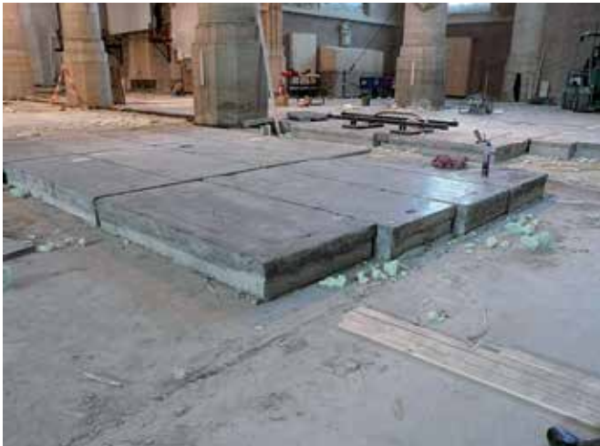
FIG. 6.7 The petit granit gravestones furnished with concrete layer to enhance thickness, lying on the special floor where the heating pipes run (Peter's church, Leiden, The Netherlands) / photo: R. v. Hees
