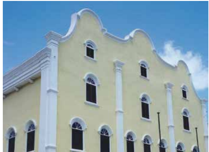
FIG. 4.8 Façade furnished with a salt resistant render system in 1994, situation 6 years later (synagogue, Curaçao, Caribbean) / photo: R. v. Hees
