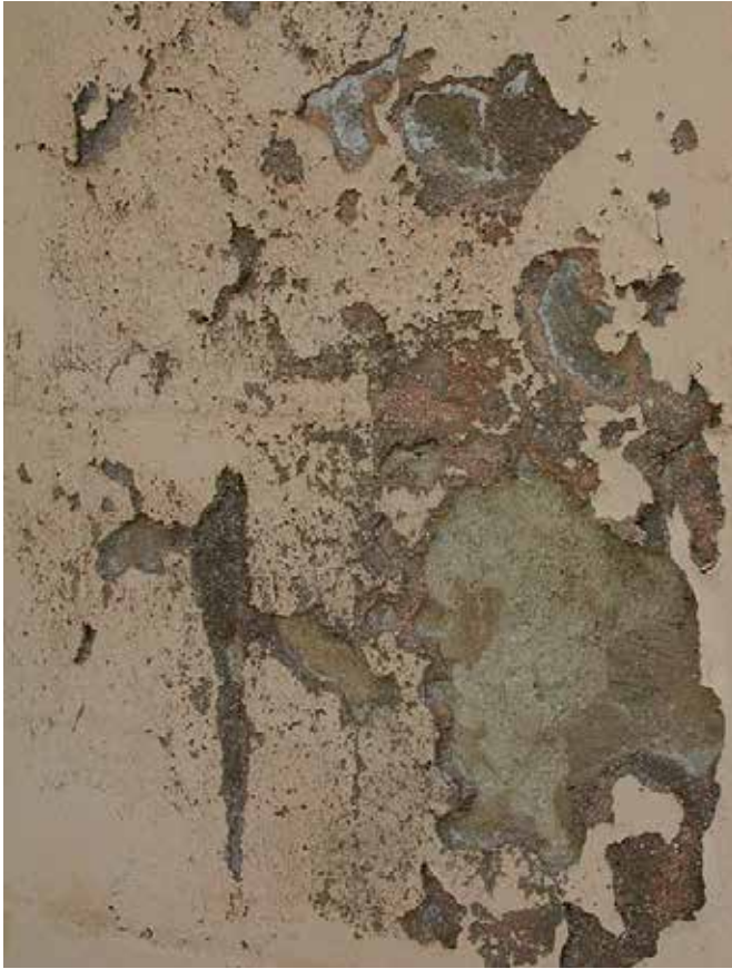
FIG. 4.5 With the use of 'better', more durable materials, sometimes damage is induced: here the plaster shows loss of cohesion (building, Curaçao, Caribbean) / photo: R.v.Hees
